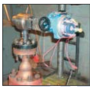
Steam Cycle Testing
